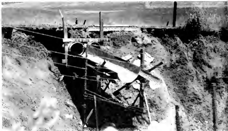
FIG. 31a. Projecting culvert with temporary extension, added after serious loss of embankment
